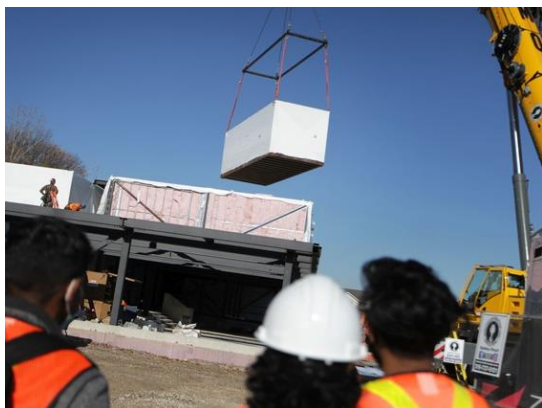
A crane hoists a prefinished modular containing a bedroom unit and a living room unit onto a new residence building at St. Clair College’s main campus on Thursday, Nov. 12, 2020. A worker guides a prefinished modular
